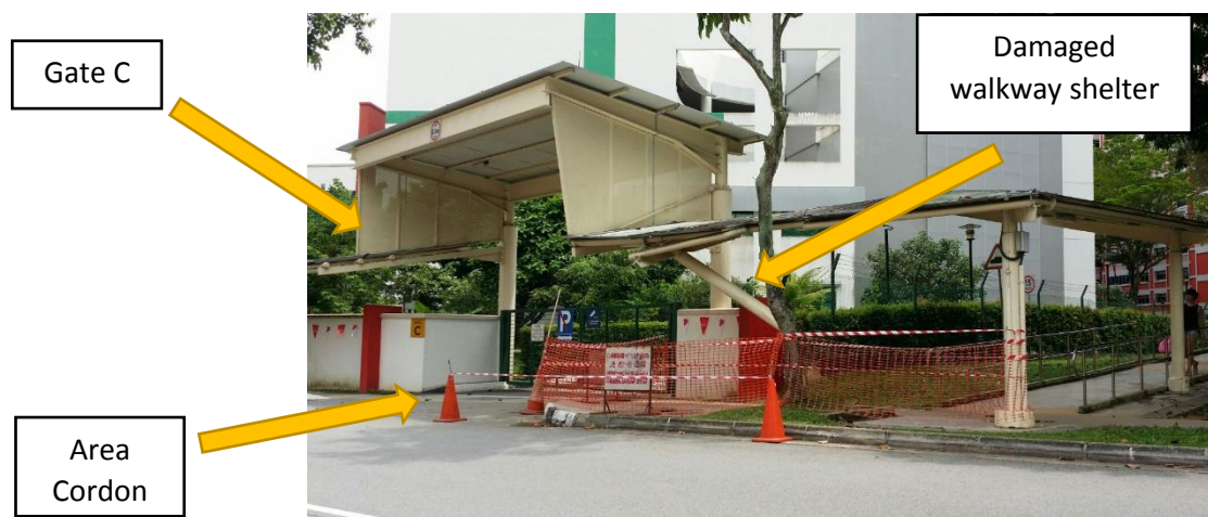
Photo 1: Accident site on Sat 30 Jul 2016
